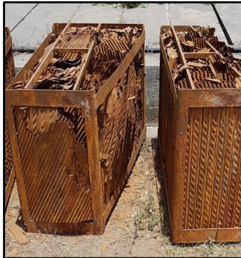
Defective APH baskets
